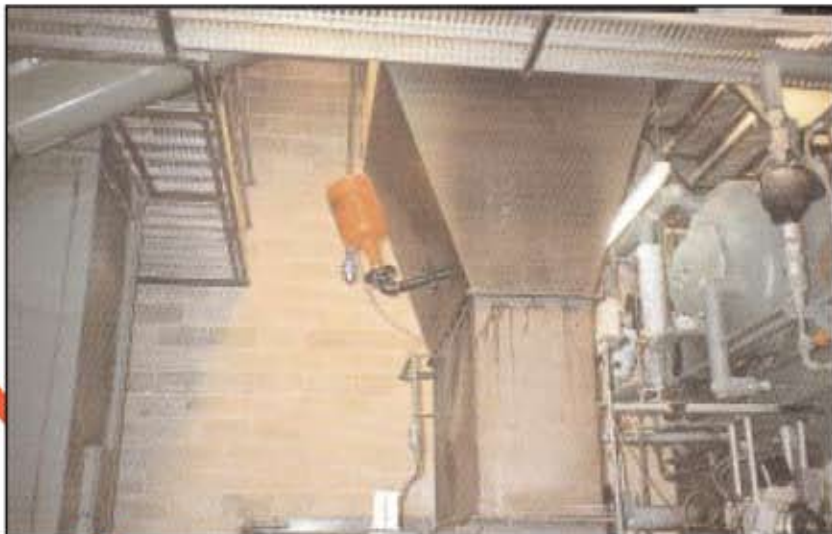
ABS-2 KEEPS WOOD CHIPS FLOWING: Air cannon was placed just above stacker chute to keep it clean and wood chips flowing. Ask for Bulletin 9124.
